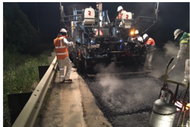
Laying asphalt in the shoulder of the Monash Freeway - works like this can be a source of noise during road construction projects.
